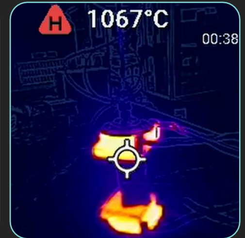
Thermal image during operations
